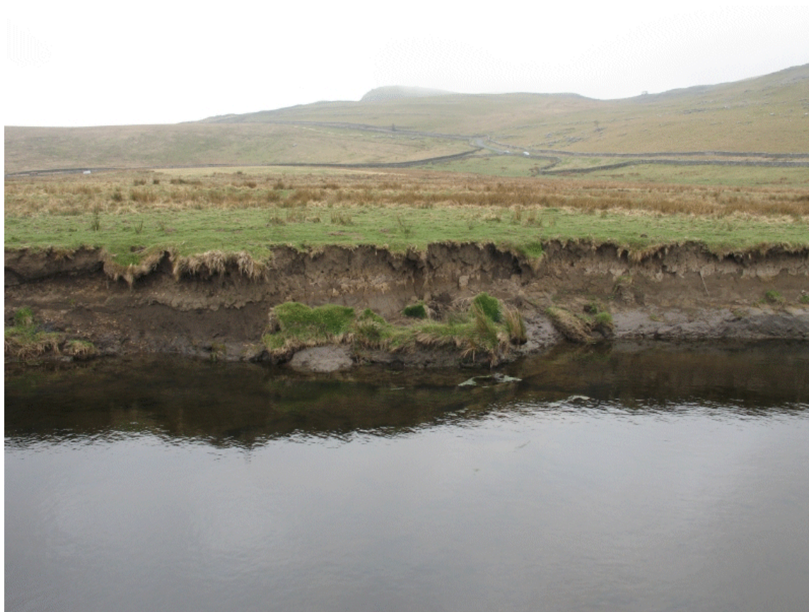
Plate 5: Sandymire – showing area of collapsed bank
